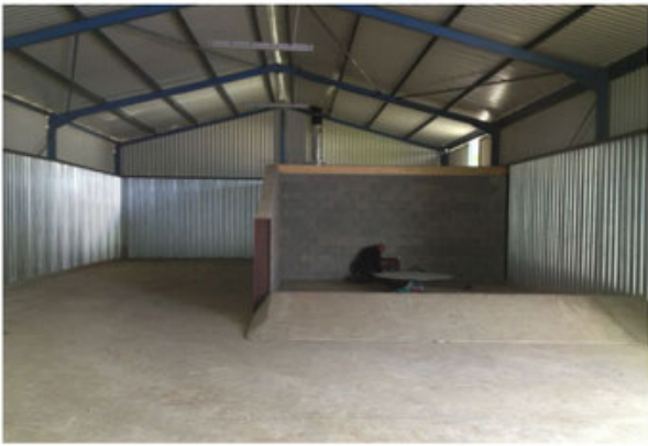
Large annual and immediate fuel store within a single building
