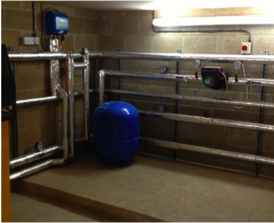
ETA Hack (70kW boiler room fully lagged and ready for operation)
