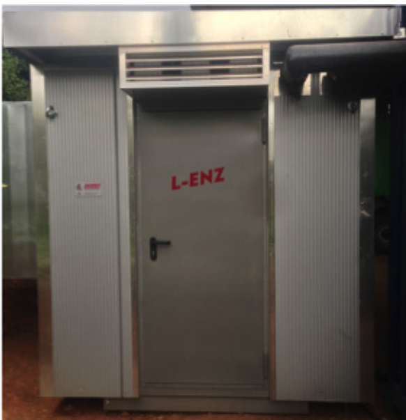
Laubler L ENZ Unit ready for operation
