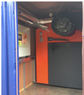
Containerised boiler (front)
