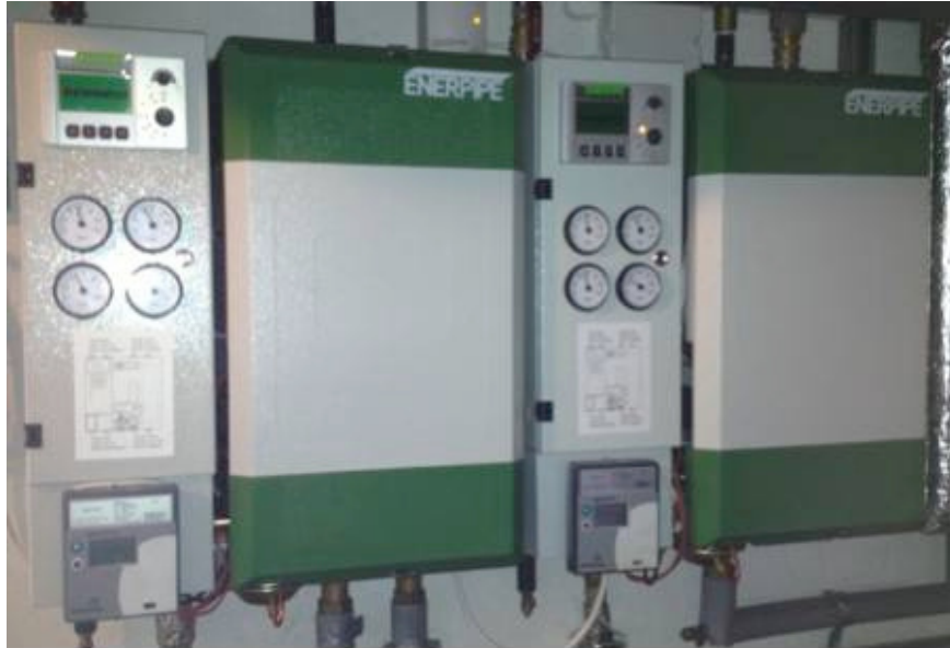
Enerpipe heat transfer units with Kamstrup Class II RHI compliant heat meters
