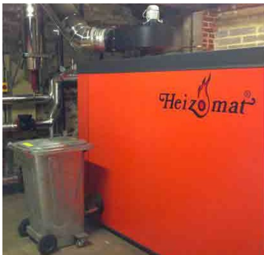
Heizomat RHK-AK 204 boiler (198kW output)
