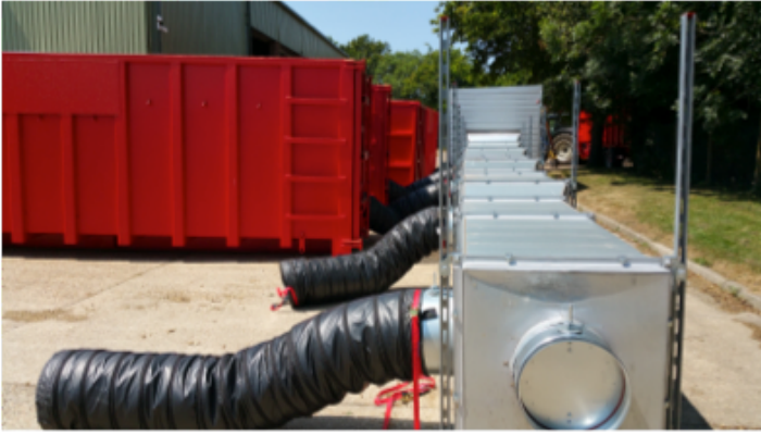
Air ducts that transport the heat from the Drying Unit to the containers of wet wood chip.
