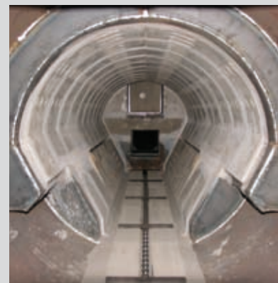
Combustion chamber with de-ashing chain.
