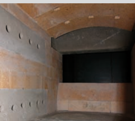
Fully fireclay lined combustion chamber.
